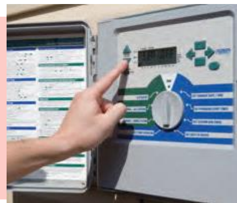
Figure 4. Adjusting a sprinkler system.
